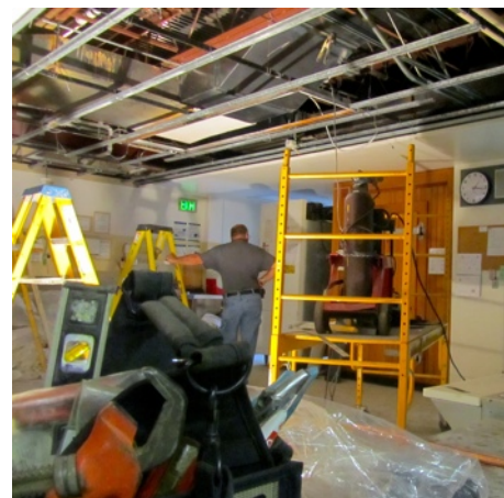
One of the unexpected results of the remodeling project was the installation of an updated fire suppression system for the kitchen, shown above.
