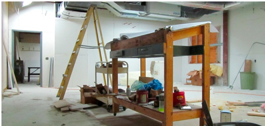
A view of the remodeling project as of late July, showing the site of the future 6th grade classroom. The door on the left and an adjacent hallway will lead to the 5th grade classroom.
